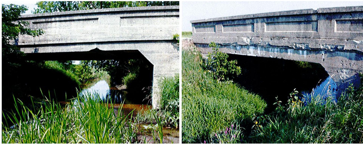
Figure 12 – CA004A (left) and CA009 (right) are concrete T-beam bridges built in 1935 over Caledonia and Paxton creeks, respectively. (Keystone, 2013)
