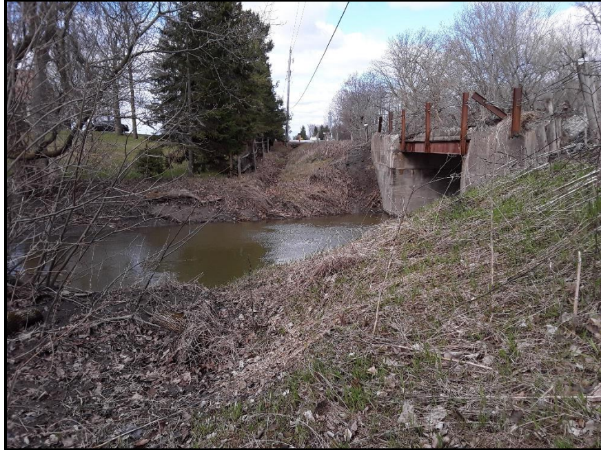
Image 3. View of the bridge which crosses Butternut Creek and associated disturbed slopes south of Paul Latour Road (Route 800), facing west. (PR21-022D014)
