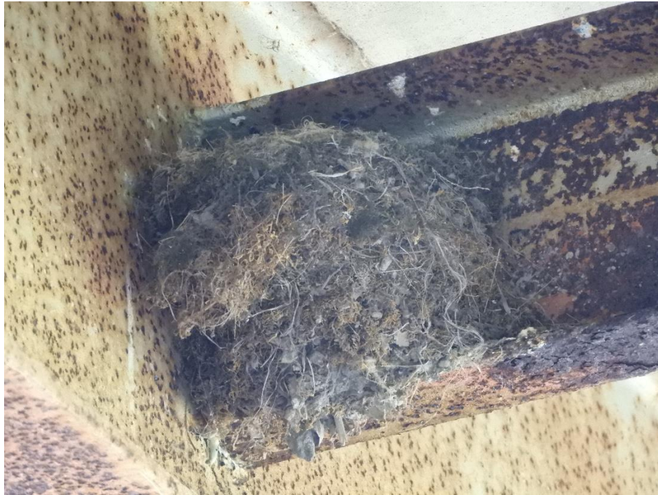
Photo 11: An active Eastern Phoebe ( Sayornis phoebe ) nest observed in the Route 800 culvert. 26 May 2021.
