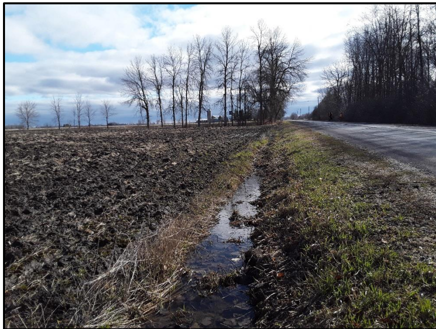
Image 4. View of the saturated culvert south of the active agricultural field, facing east. (PR21-022D005)
