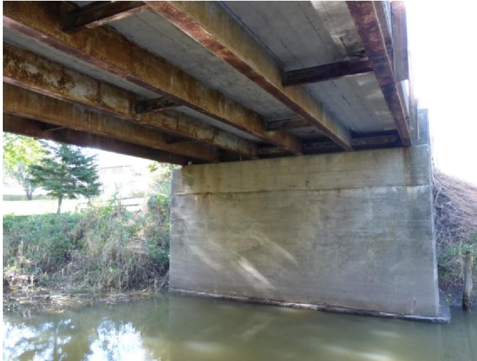
Figure 5 – The steel girders sit on concrete abutments, and the reinforced concrete deck is laid over the girders. (LSHC 2013) 042
