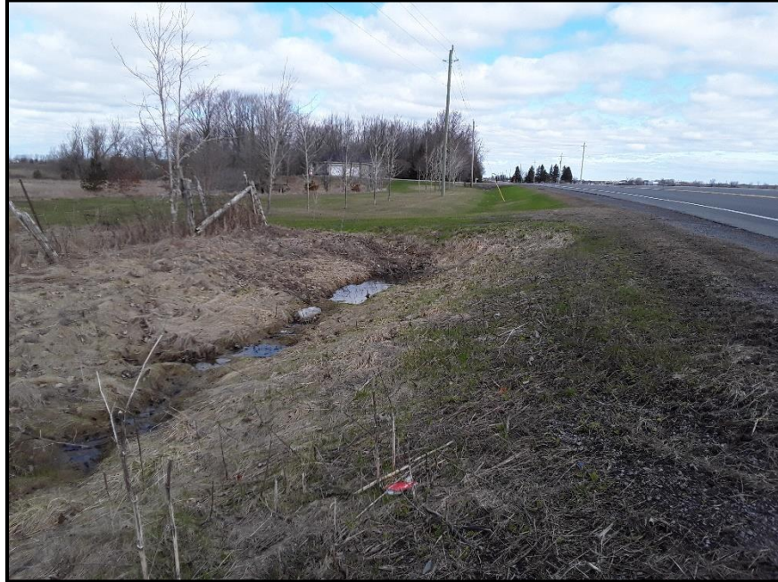
Image 5. View of the saturated culvert west of County Road 7, facing north. (PR21-022D018)
