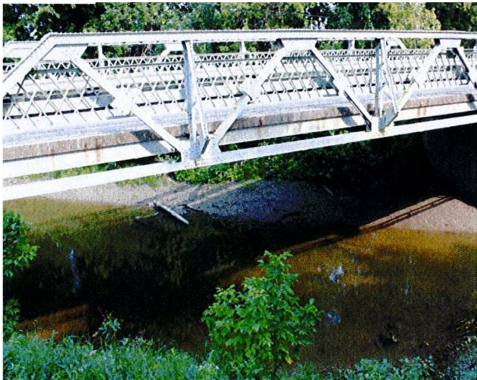
Figure 10 – SP010 “Wilson Bridge”, is a pony-truss bridge built in 1919 over the Scotch River. (Keystone, 2013)
