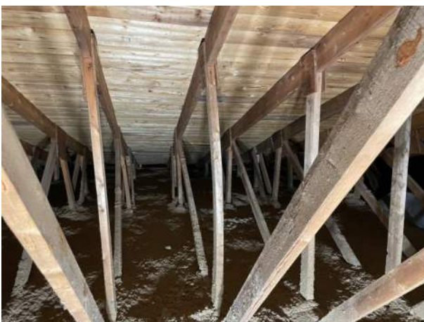
Photo #11: Swaying/Bending Truss Members
