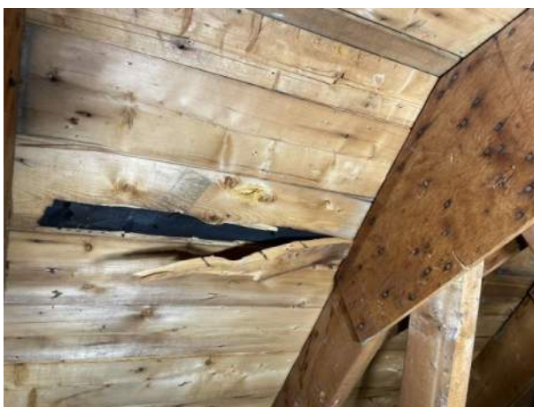
Figure 3: Localized Roof Sheathing Damage
