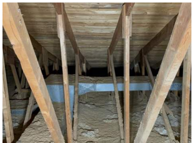
Photo #12: Swaying/Bending Truss Members
